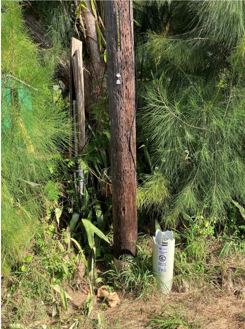
There is an ATT buried cable of unknown direction in the alley in the area of the west end of the property.
