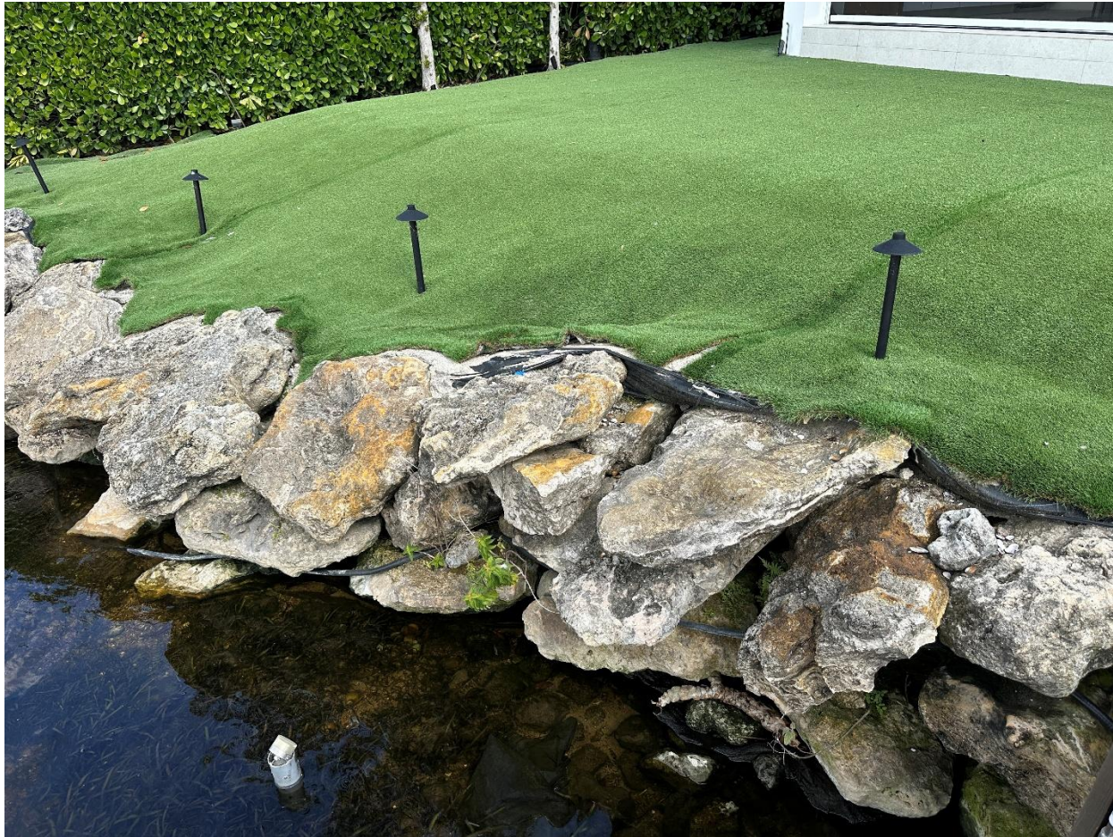
NORTH END ROCK WALL – ELEVATION 8.91' SINKHOLES VERY AGGRESSIVE SLOPE
