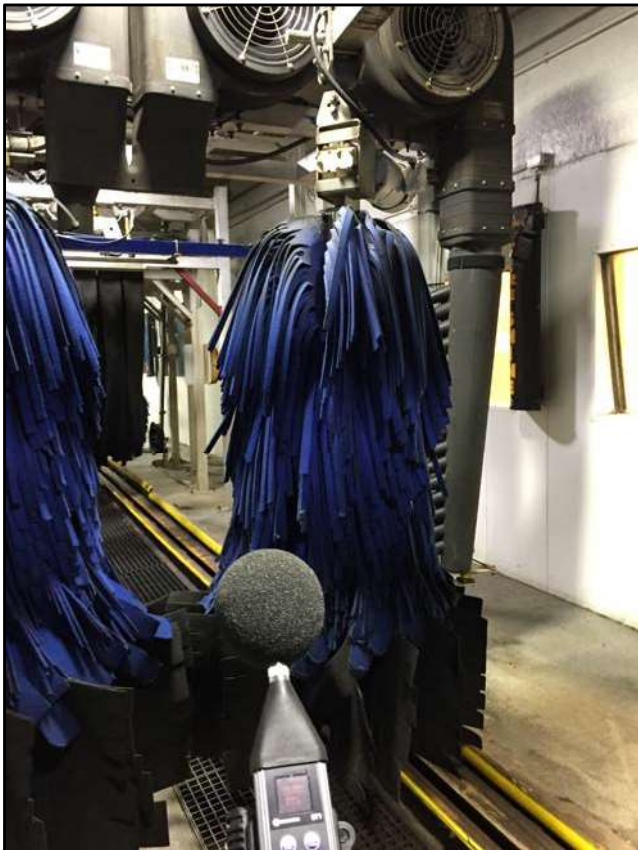
Photo 3. Dryer Blowers Without Silencers
